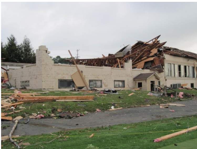
Tornado Damage to Buildings in Chautauqua County
